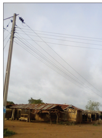
Plate 1: Electricity lines not connected to Grid at Alabi village (Ibarapa North local government area)
