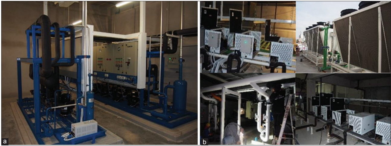
Figure 8: Those are elements of 2 types of refrigeration system: (a) Conventional multi set rack (b) Water loop system
